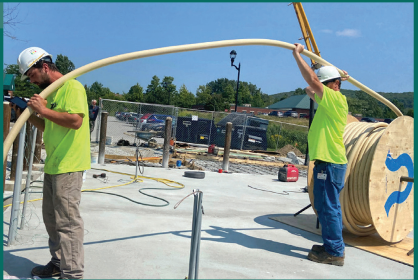
Oxygen main line for medical center.
