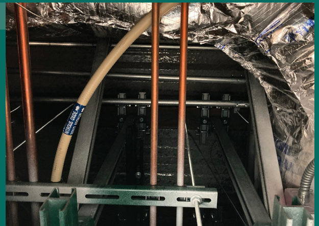
MediTrac® CMT installed above a finished operating room ceiling.
